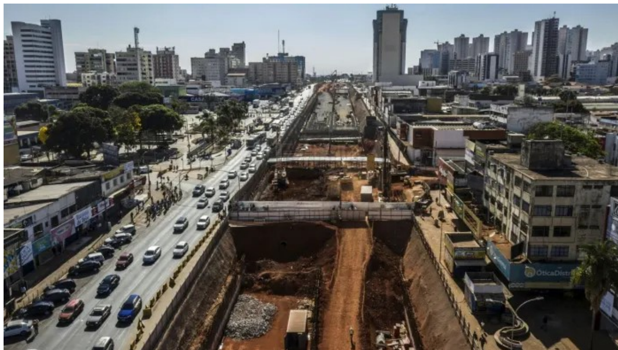
An express underpass road under construction in Tabatinga, Brazil. The country's economy grew more than 6% a year from 1951-80 © Dado Galdieri/Bloomberg
