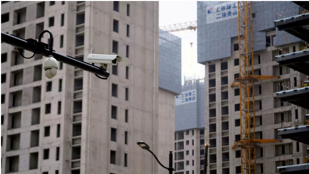
Residential buildings under construction in Shanghai. The property market has seen waves of defaults among developers and a fall in transactions © Aly Song/Reuters
