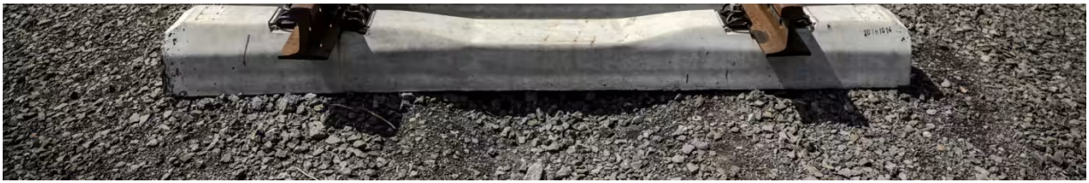
Incomplete rail tracks for the Standard Gauge Railway line lay on the ground near Duka Moja, Kenya © Luis Tato/Bloomberg
