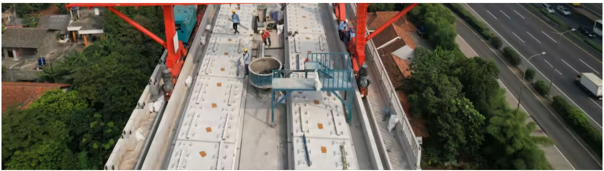
The construction of an elevated track for the Jakarta-Bandung high-speed railway in Cikarang, West Java, last month © Dimas Ardian/Bloomberg
