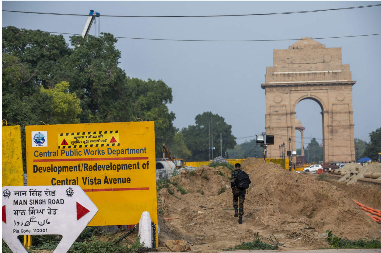
A security worker walks through a construction site at Kartavya Path, formerly Rajpath, on the Central Vista, in New Delhi. Photograph by Prashanth Vishwanathan / Bloomberg / Getty
