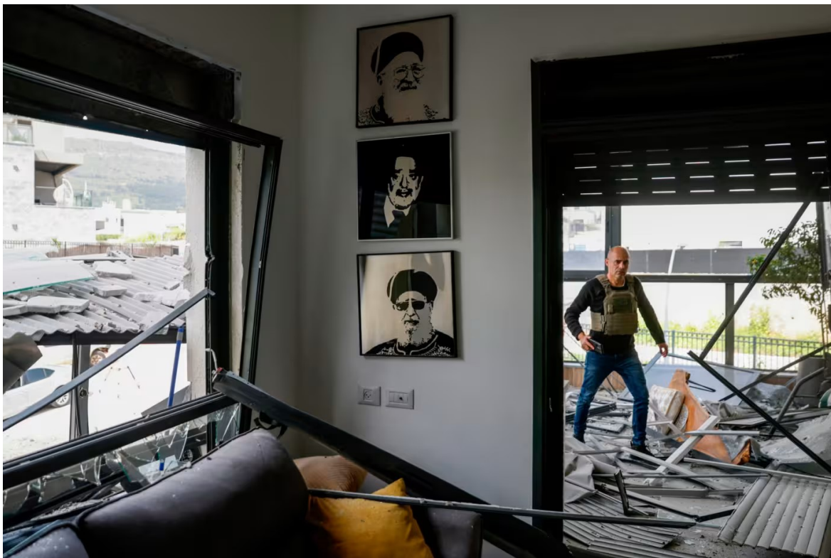
A man inspects a damaged home in Kiryat Shmona, northern Israel, after it was hit by a Hizbollah rocket on Wednesday © Jalaa Marey/AFP/Getty Images
