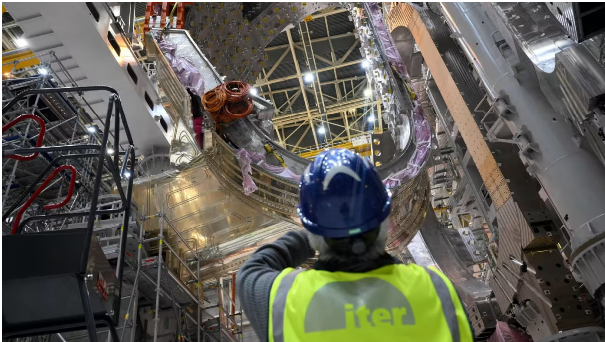
A module being assembled at the Iter nuclear fusion project in Saint-Paul-les-Durance, southern France © Nicolas Tucat/AFP via Getty Images
