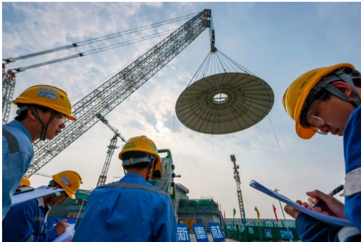
Construction of the Changjiang nuclear reactor in Hainan, China's southernmost province. China is building nuclear power plants to reduce its reliance on coal © China News Service via Getty Images
