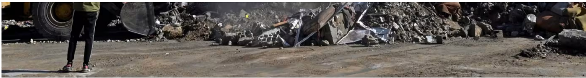
Diggers clear debris from destroyed buildings in Nabatiyeh, southern Lebanon © Wael Hamzeh/EPA-EFE/Shutterstock
