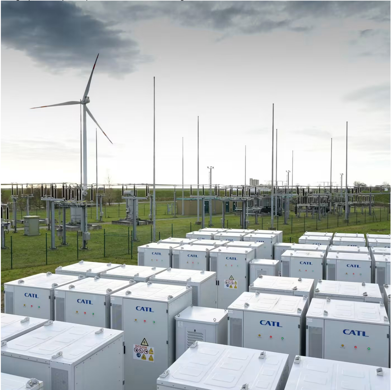
A wind farm with battery storage facilities made by CATL in Germany. There have been concerns in Europe of excessive reliance on imports from China © Alamy
